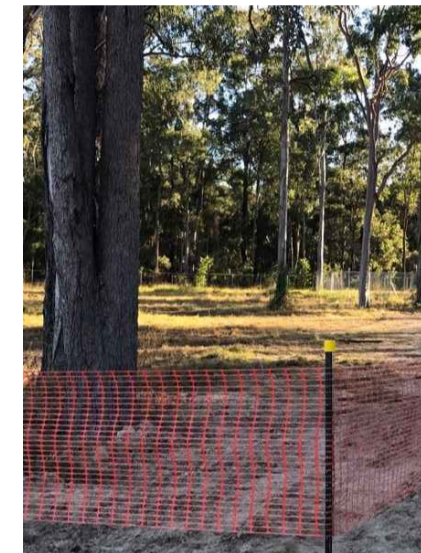
04 FIGURE 4 TPF2 VM08 Orange mesh with steel staking to be used in support locations and where ground conditions limit the access for TPF1. Fence line to be based on surveyed positioning.
