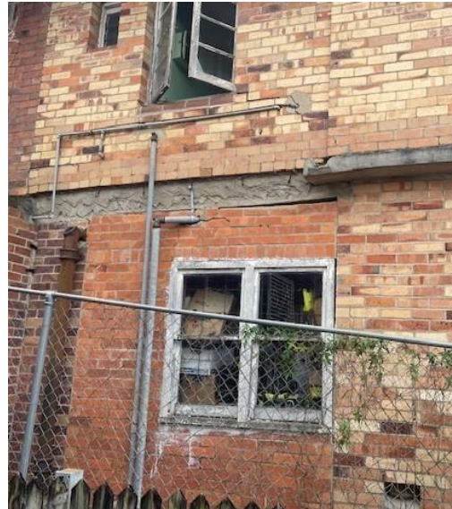
Figure 11: Structural damage to brick addition
