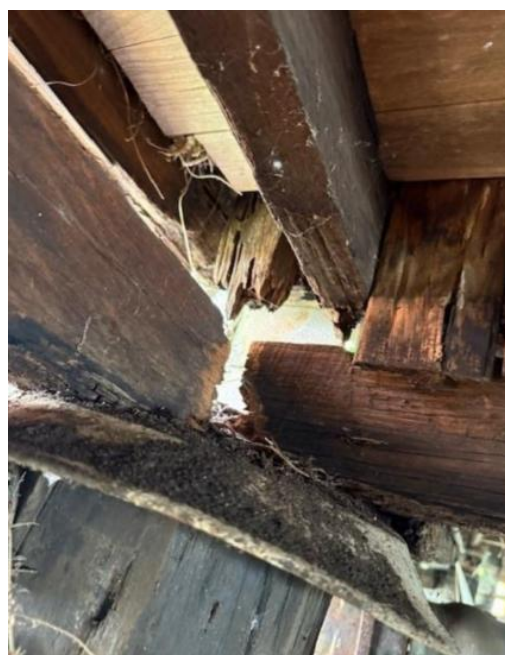
Figure 9: Stumps disconnected from floor joists
