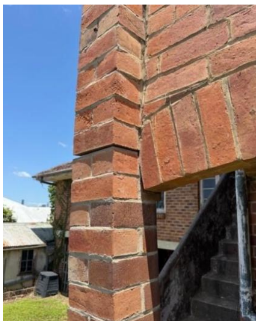
Figure 15: Exterior brick columns failing
