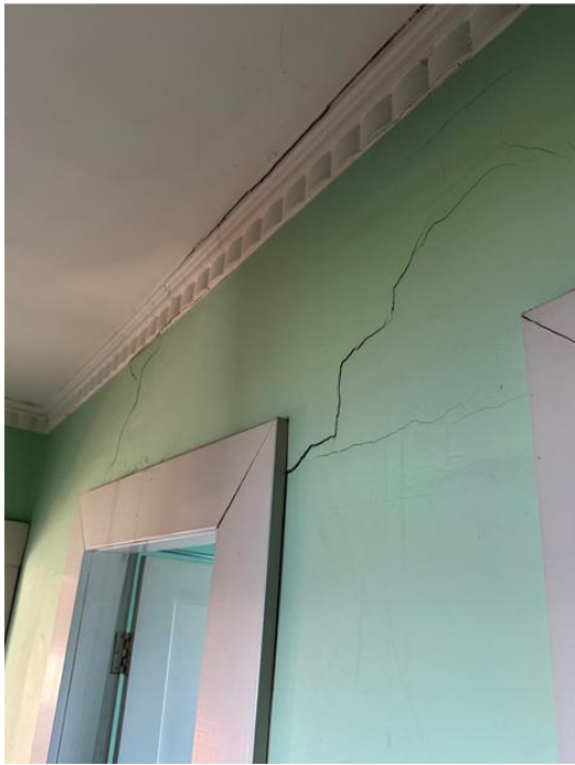
Figure 16: Internal Structural Damage
