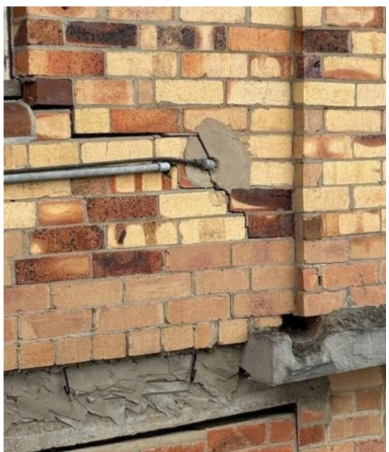
Figure 14: Structural damage to brick addition
