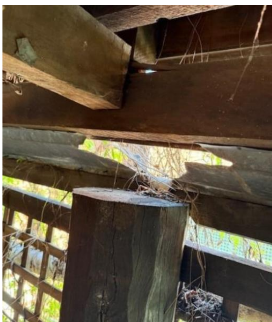
Figure 8: Stumps disconnected from floor joists
