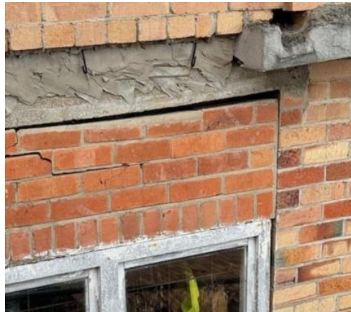
Figure 13: Structural damage to brick addition
