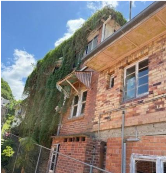
Figure 10: Vegetation attached to timber cladding
