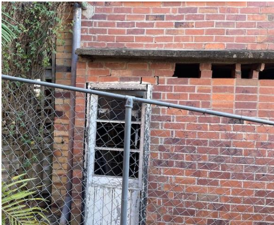
Figure 12: Structural damage to brick addition
