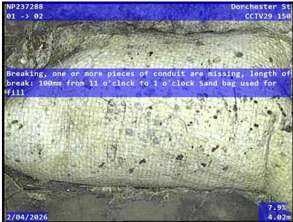
7, 00:02:01, 4.02 Breaking, one or more pieces of conduit are missing, length of break: 100mm from 11 o'clock to 1 o'clock / Sand bag used for
