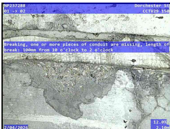
5, 00:01:13, 2.10 Breaking, one or more pieces of conduit are missing, length of break: 100mm from 10 o'clock to 2 o'clock
