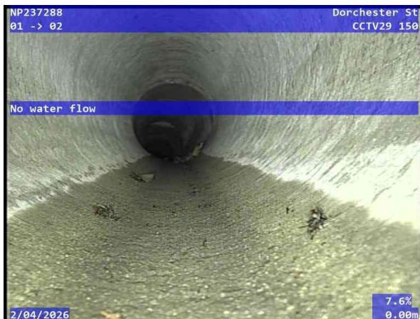
3, 00:00:21, 0.00 No water flow
