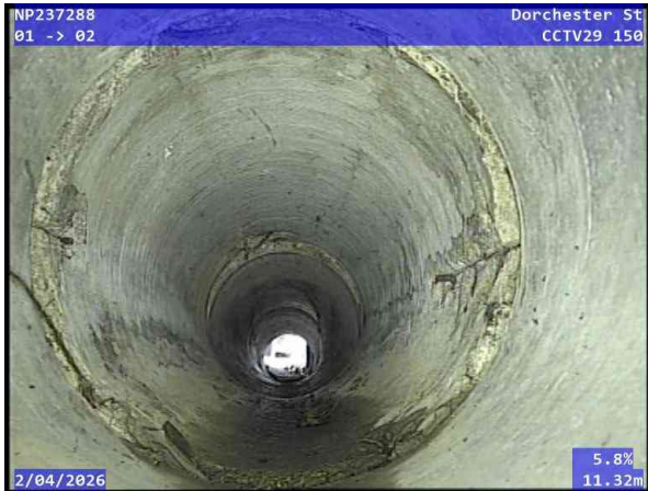
13, 00:05:00, 11.32 Breaking, one or more pieces of conduit are missing, length of break: 100mm from 11 o'clock to 1 o'clock / Exposed rio
