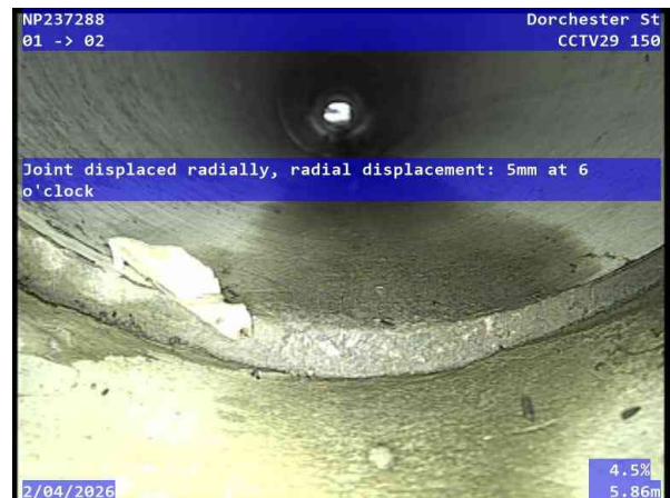
10, 00:03:28, 5.86 Joint displaced radially, radial displacement: 5mm at 6 o'clock
