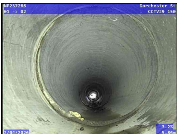
11, 00:03:28, 5.86 Joint displaced radially, radial displacement: 5mm at 6 o'clock
