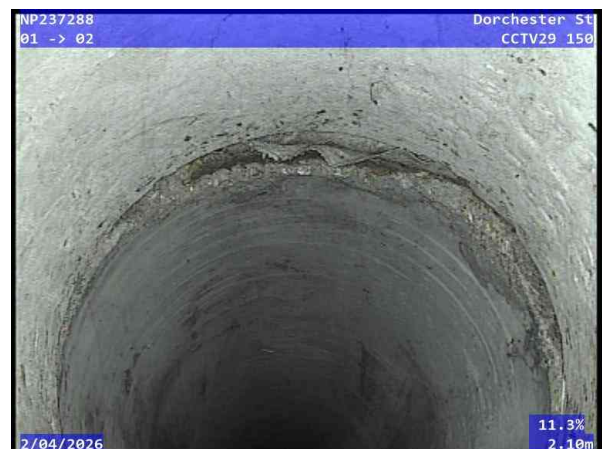
6, 00:01:13, 2.10 Breaking, one or more pieces of conduit are missing, length of break: 100mm from 10 o'clock to 2 o'clock
