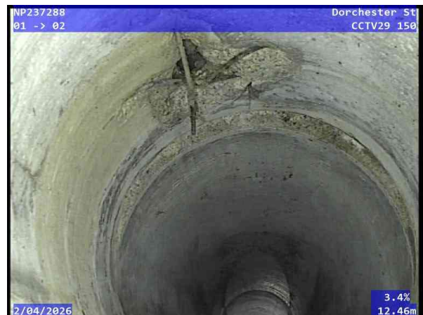
16, 00:06:01, 12.46 Void visible through defect
