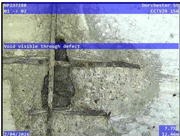
15, 00:06:01, 12.46 Void visible through defect
