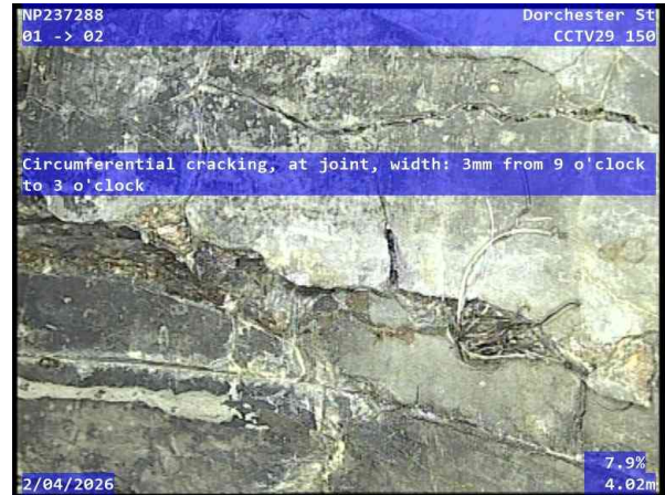
8, 00:02:10, 4.02 Circumferential cracking, at joint, width: 3mm from 9 o'clock to 3 o'clock
