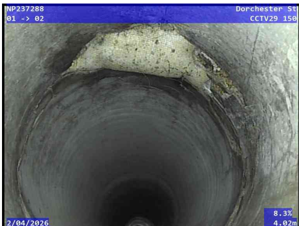
9, 00:02:10, 4.02 Circumferential cracking, at joint, width: 3mm from 9 o'clock to 3 o'clock
