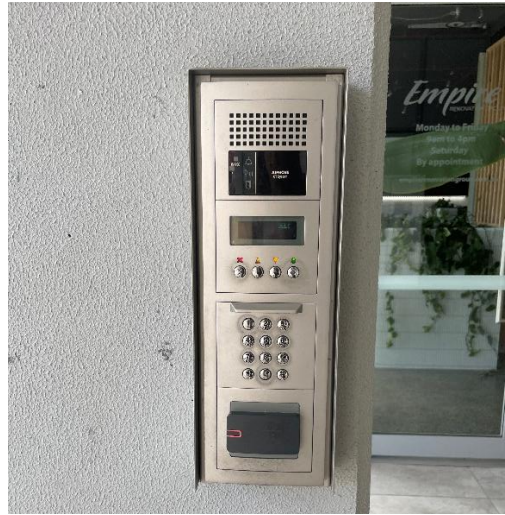
Intercom on Pedestrian Walkthrough
