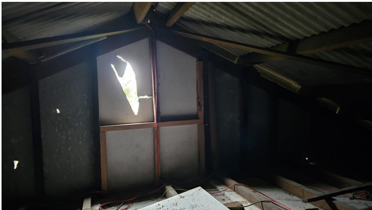
Photo 7: Gable End Wall – Damage Wall Cladding
