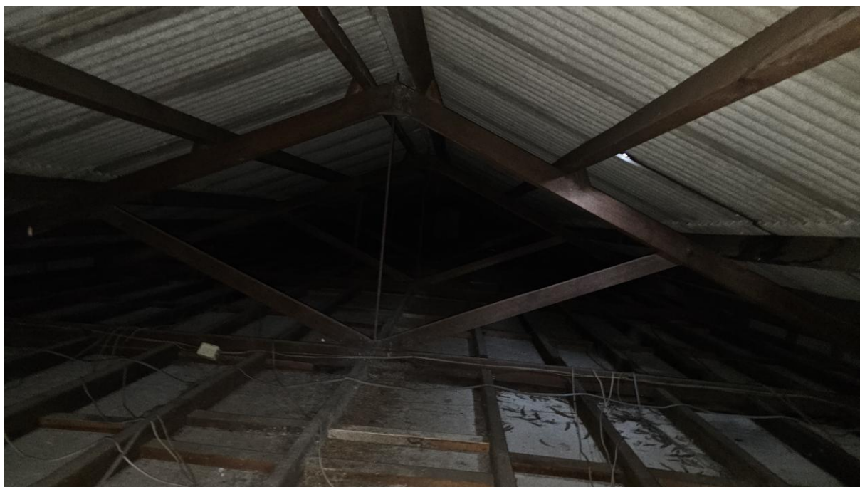
Photo 8: Roof Framing – Damaged Roof Sheeting
