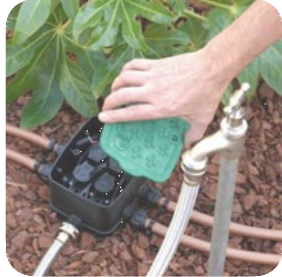
IRRIGATION Drip line irrigation system to be fully automated to cover all planter garden areas, with environmentally reactive controller (HYDRAWISE pro-FC controller or like product) to maintain plant health in extreme conditions 90mm PVC conduit pipe under slab/pavement for irrigation/electrical access to all garden beds
