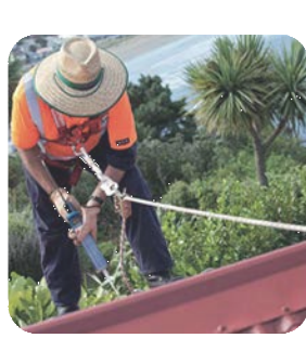
4 MAINTENANCE SAFETY Balcony planter and roof top planter maintenance must utilise 'anchor and harness' style fall protection systems (XSPlatforms 'LinkdPro' or like product)
