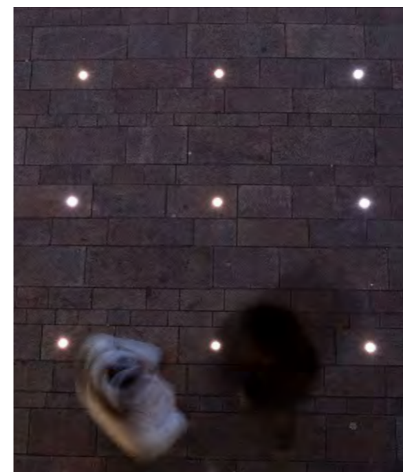
LED Up-light within paving
