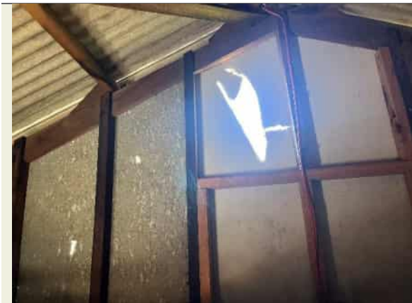
Figure 8-1: Damage to external cladding in roof void
