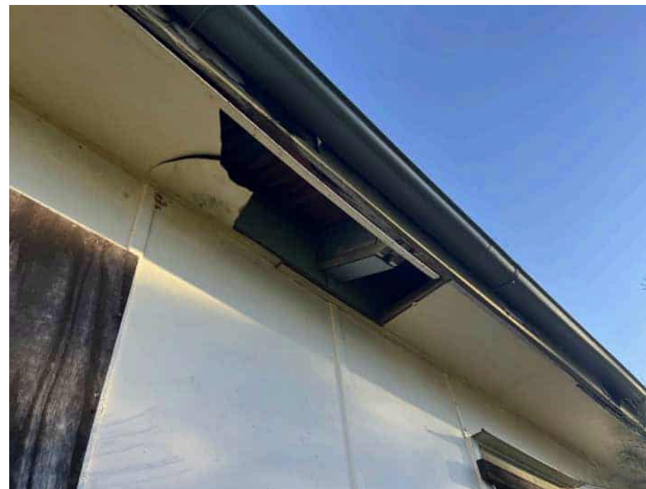
Damage to soffit sheeting
