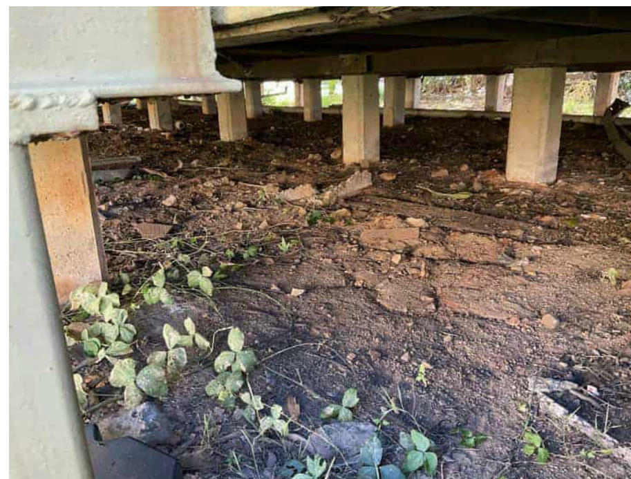
ACM debris below building
