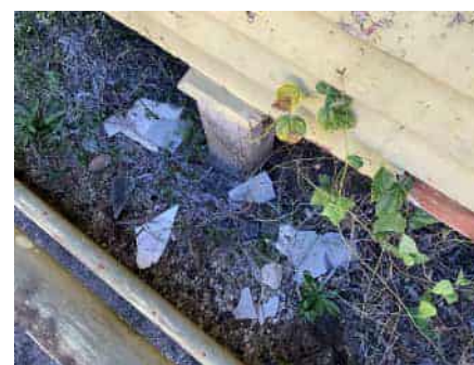
ACM Debris adjacent building
