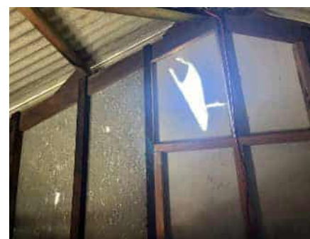
Debris in roof void presumed due to damage to external cladding
