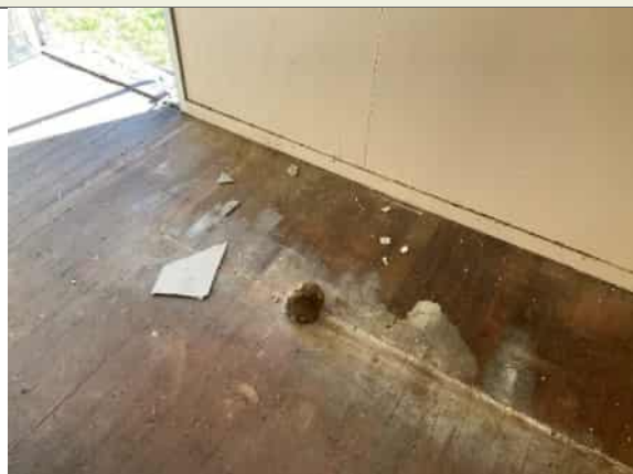
Figure 8-3: Debris from external cladding damage
