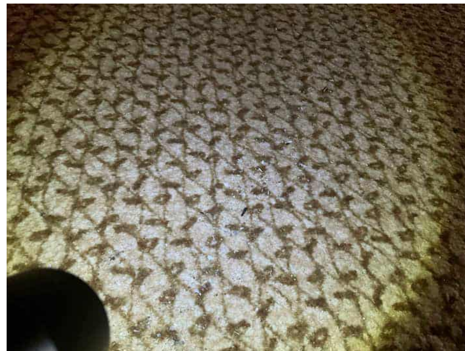
Debris on ground from damage to linings
