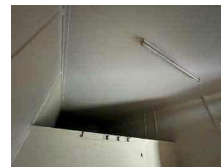
Shower rom ceiling
