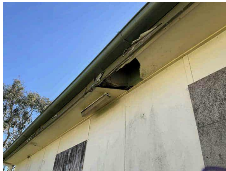
Damage to soffit lining
