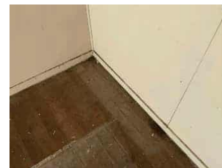
ACM debris on ground
