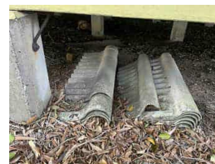
Stored ACM roof sheeting below building
