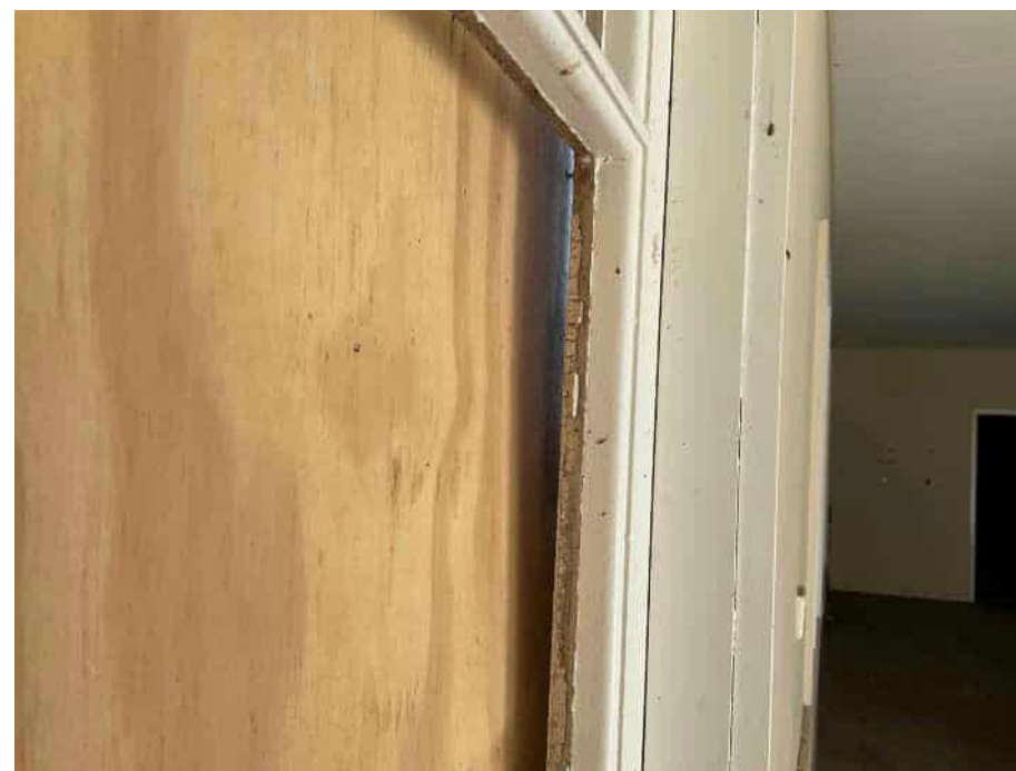
Northwest and northeast rooms window putty
