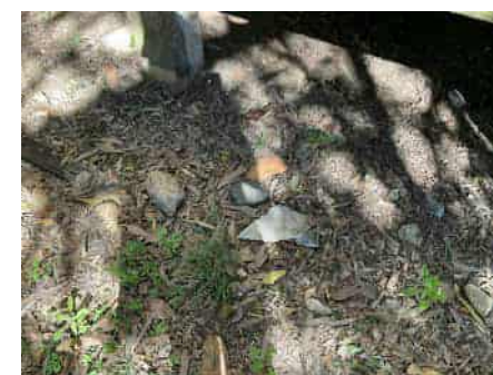
ACM Debris adjacent building
