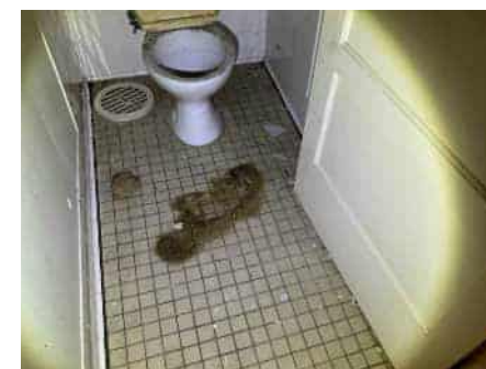
Debris on ground from damage to linings
