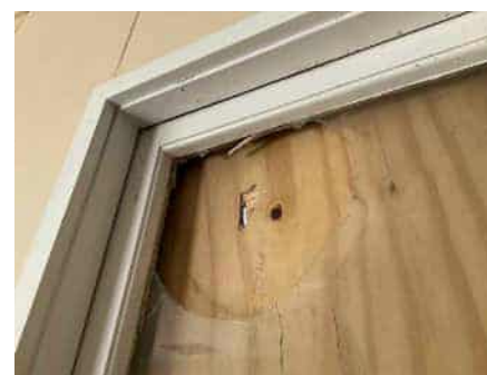
Northwest and northeast rooms window putty
