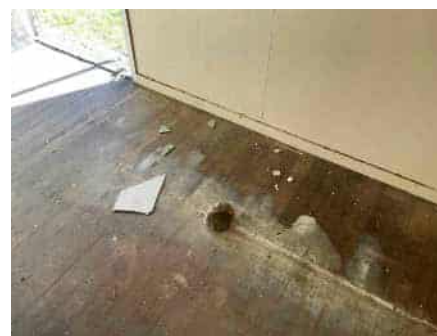
ACM debris on ground
