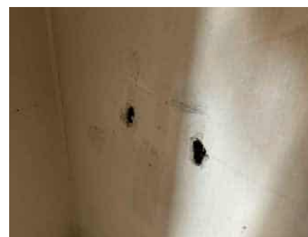
Damage to partition/ cubicle walls
