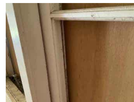
Northwest and northeast rooms window putty
