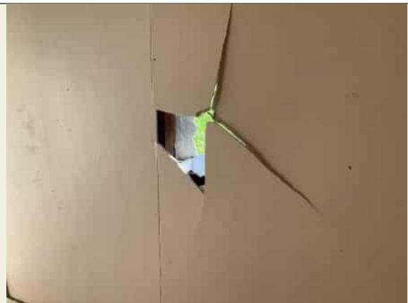
Figure 8-2: Damage to external cladding coming into internals
