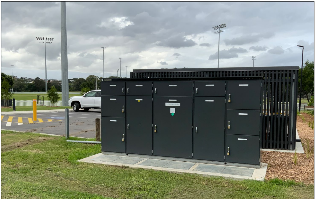
Figure 9 – Existing main switchboard (Source: Indara 2023).
