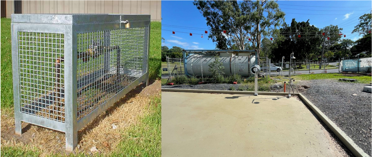
Figure 7: Hose reel, safety shower, RPZ devices.
