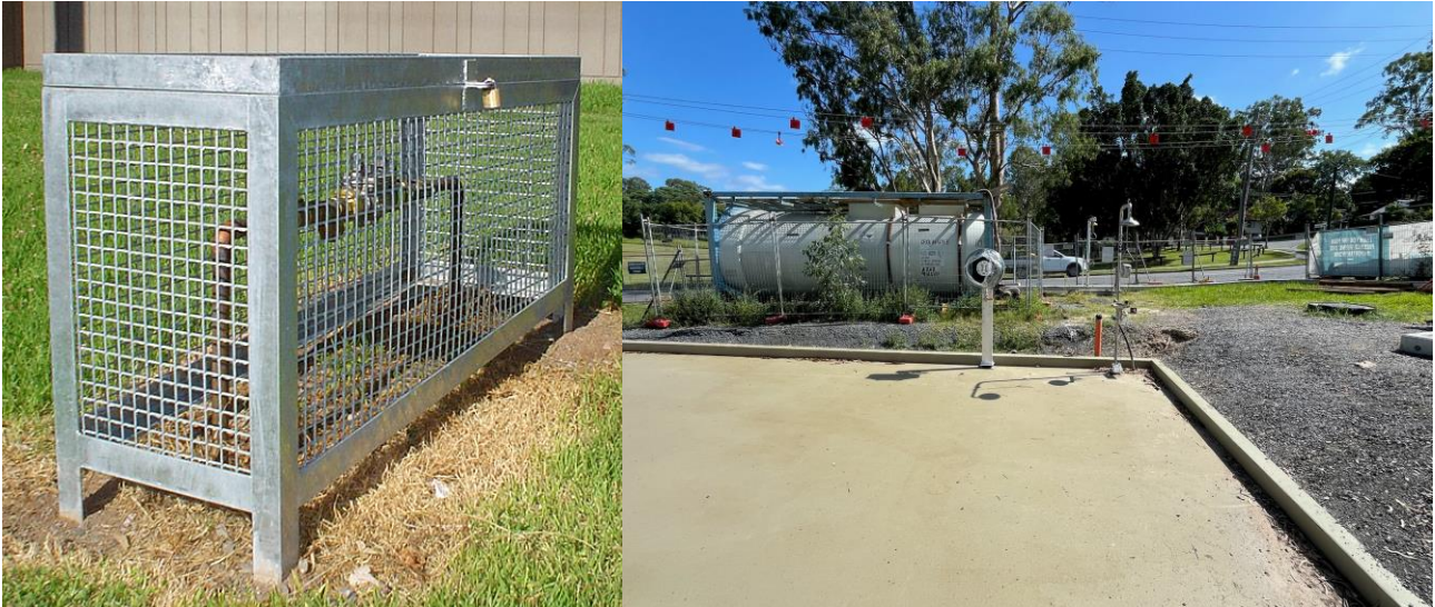
Figure 7: Hose reel, safety shower, RPZ devices.
