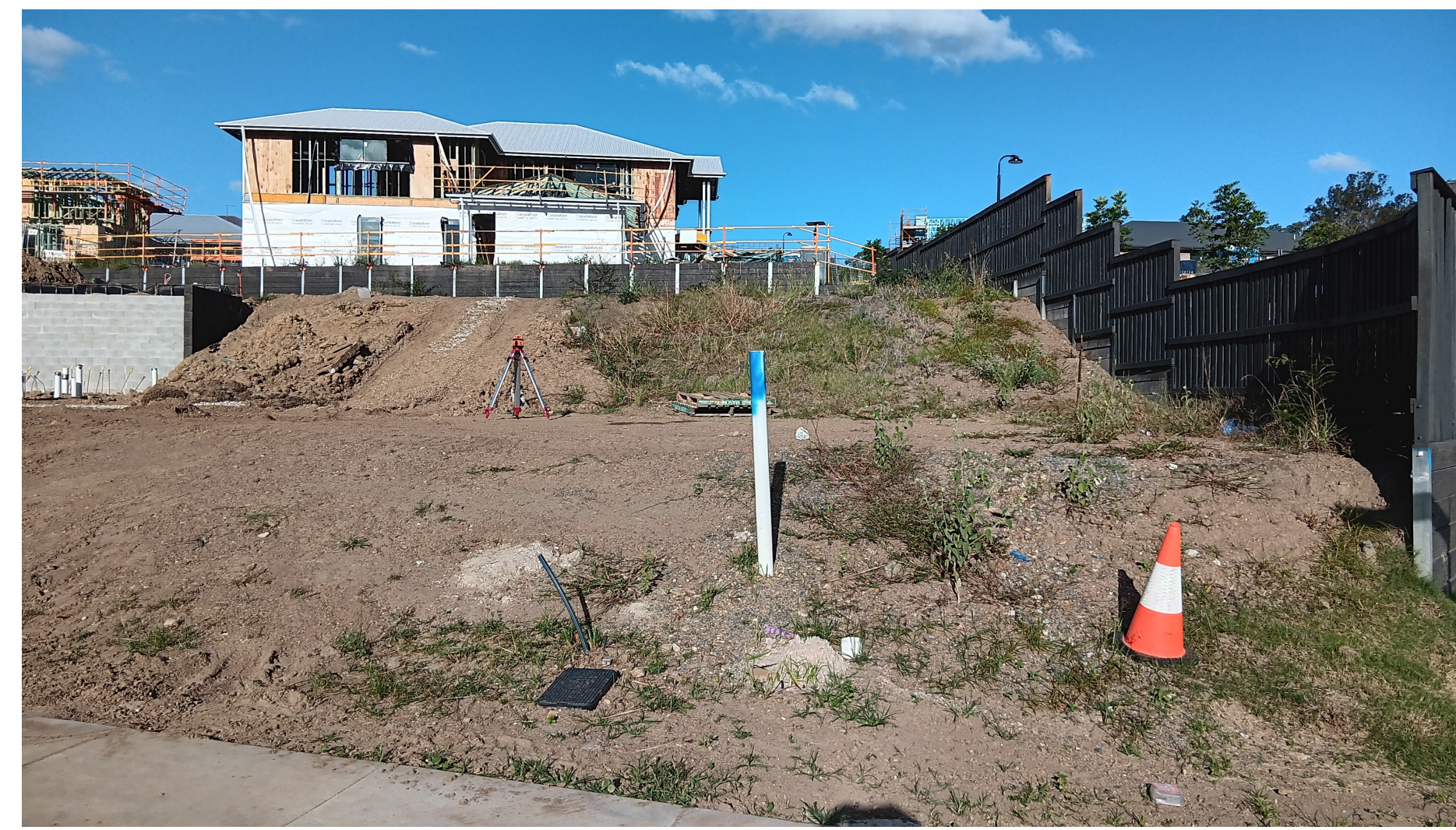
Photo from Halifax Street Looking up the block. Large retainer wall and fencing along Holbourne Street Visibly. Retainer wall and fencing as per Developer's approved BCC DA
