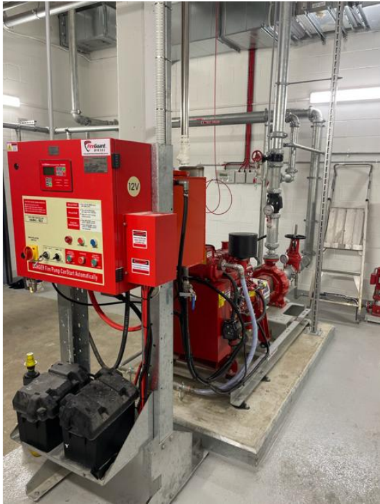
Figure 3 – Photo of fire pumps, diesel engines and fuel tanks
