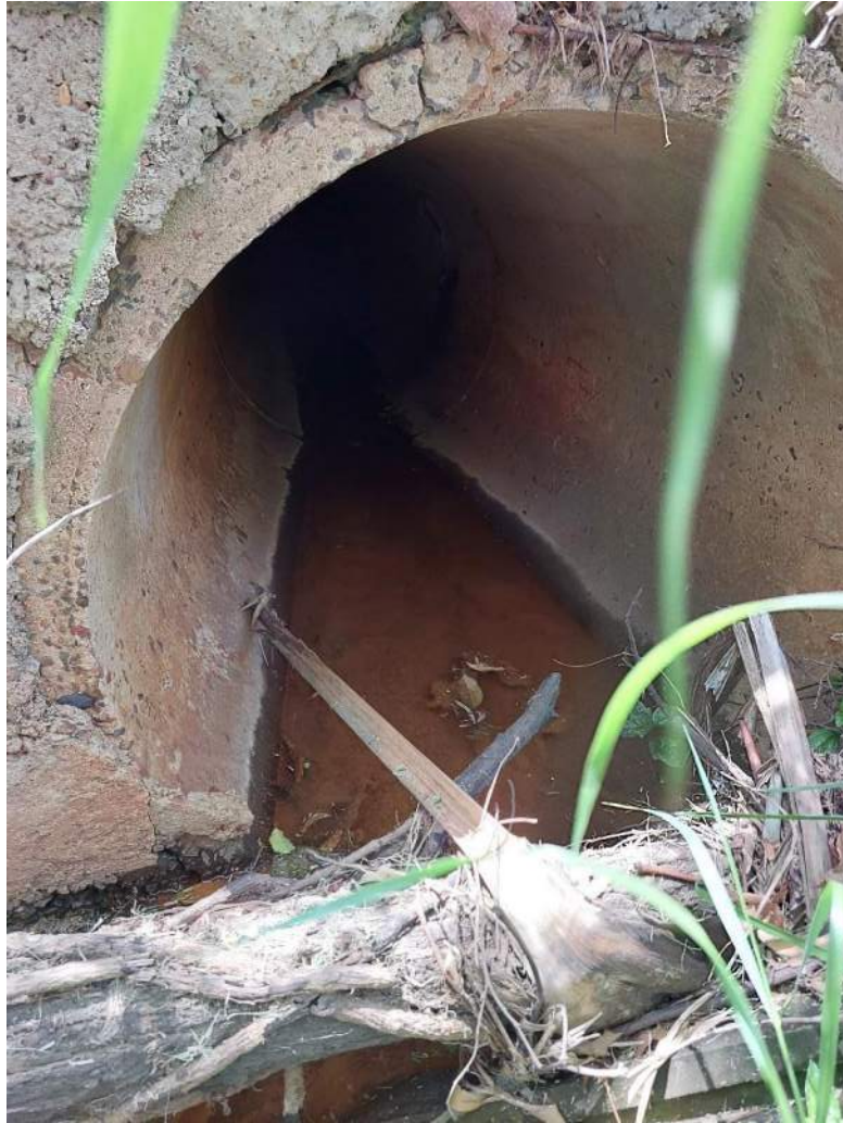
Figure 5 – 900mm Diameter RCP – north-west of site (Source: MPN Site Visit)
