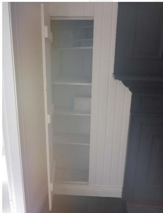
Figure 38: The wall plane beside the fireplace shown in the preceding image incorporates a discreet cupboard door that provides access into a small storage cupboard setting to the wall cavity. (Source: VAULT)
