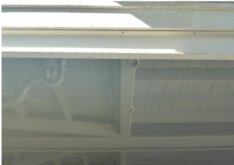
Figure 14: The view into the undercroft space situated immediately below the rear corner of the subject building; as per the preceding image. Note the differential between the sub-floor framing and decking / boarding over same between the solid core of the house (at image right) and the subsequently enclosed side verandah (at image left). (Source: VAULT)
