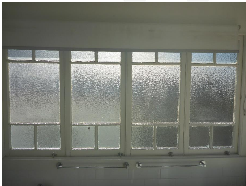
Figure 52: A detailed view of the array of four (4) multi-paned casement windows set within the bathroom space of Unit 1 and set in the side return wall of the verandah enclosure. (Source: VAULT)
