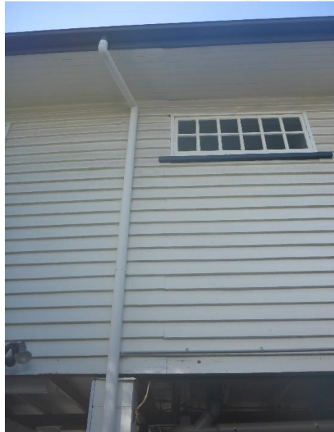
Figure 7: A more detailed view of the high-set, awning window set into the southern (side) elevation of the subject heritage residential building. (Source: VAULT)
