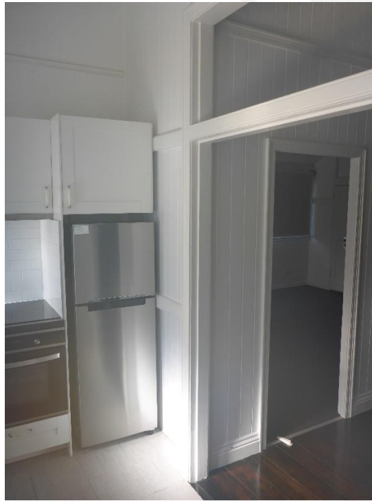
Figure 49: Another interior view from the kitchen space within Unit 1 looking back into the core of the heritage residence and showing the remnant framework of a removed French door assembly and the view through to the bedroom space within that tenancy (in background at image right). (Source: VAULT)
