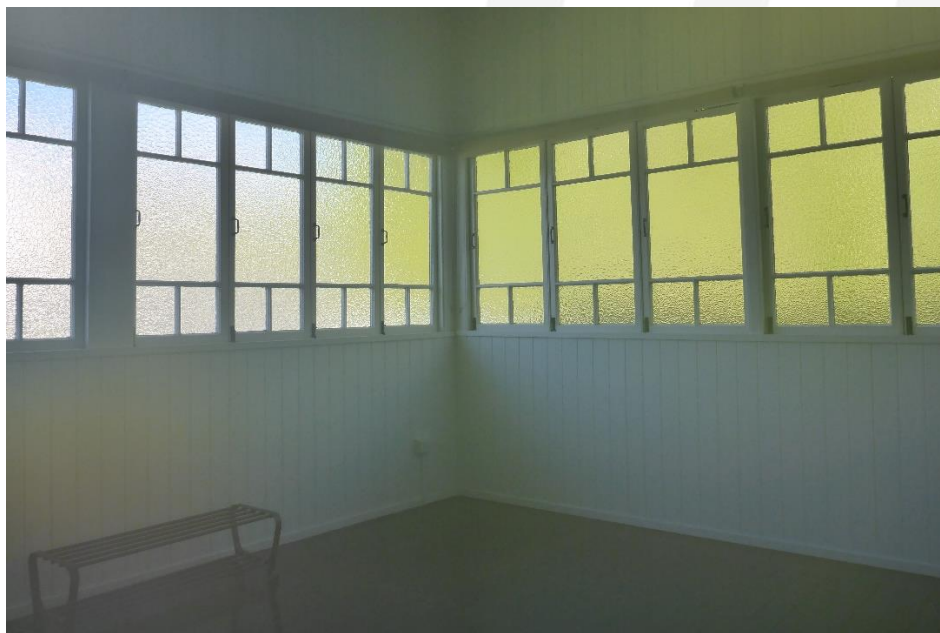
Figure 56: The reverse interior view within the bedroom space of Unit 2, which shows the array of multi-paned casement windows that now enclose this former verandah space and that extend across the front (street) elevation (image left) and extend down the side elevation (image right). (Source: VAULT)
