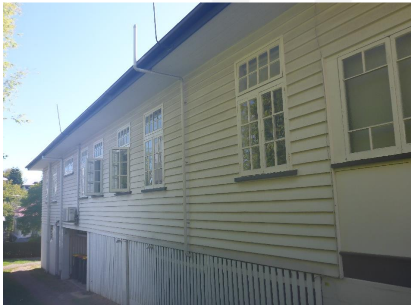
Figure 6: The view down the southern side elevation of the subject heritage building looking rearwards from the return end of the verandah enclosure (at image far right) and showing the array of original windows set into this weatherboard-clad façade of the building. (Source: VAULT)
