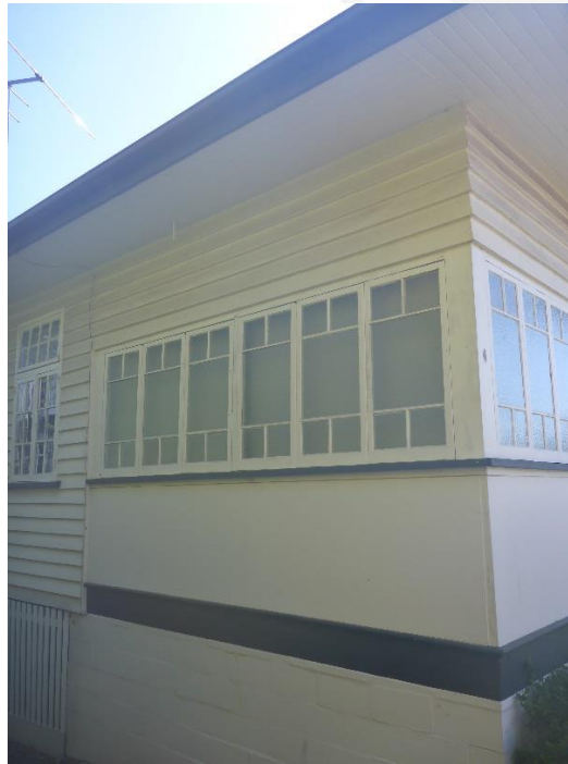
Figure 5: A detailed view of the south-eastern (front) corner of the subject heritage residential building showing how the original open verandah space has been subsequently enclosed with a combination of sheet asbestos balustrade cladding with an array of multi-paned, casement windows over. (Source: VAULT)
