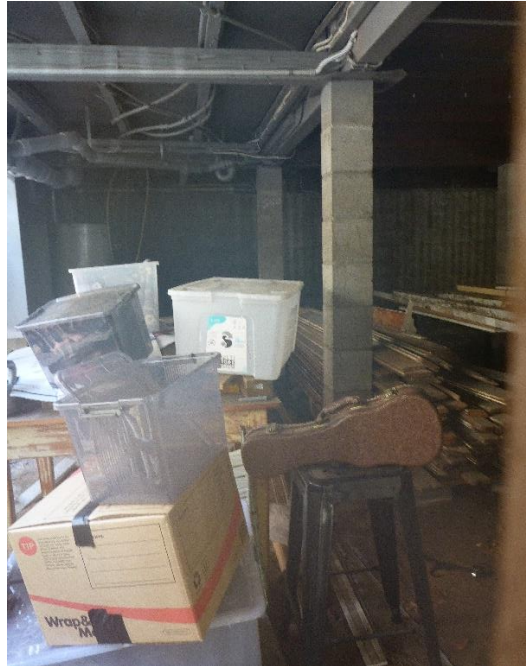
Figure 69: Another view through a different portion of the undercroft space beneath the heritage building showing how some of the supporting columns have been constructed from a vertical stack of concrete blocks. (Source: VAULT)
