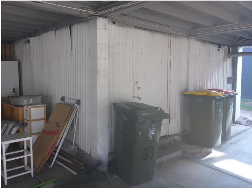
Figure 71: The undercroft space beneath the heritage building also incorporates a “lock up” enclosure that has been formed up within a series of the non-original concrete blockwork columns and has been clad in recycled corrugated iron sheeting. (Source: VAULT)
