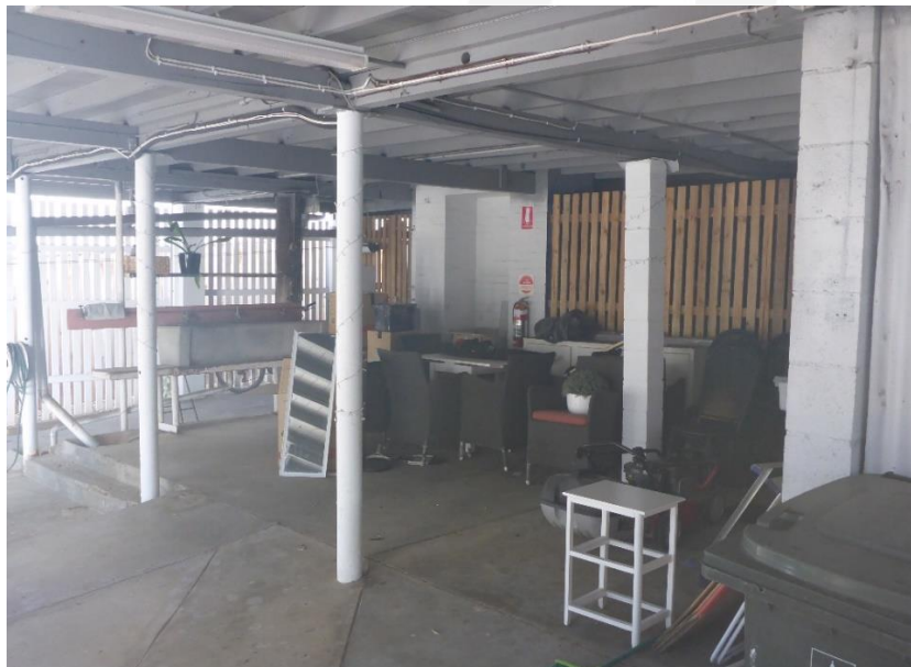
Figure 76: The reverse view across the extant undercroft space beneath the heritage building – taken from the opposite end of this space to that shown above in Figure 68 , which again shows the varied array of non-original support structures (i.e. steel posts or concrete blockwork columns) that are extant within this space. (Source: VAULT)
