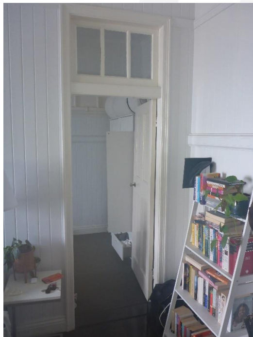
Figure 62: A detailed view of the original doorway and top light assembly situated within the partition wall between the living and bedroom spaces within Unit 4; as viewed from the living space. (Source: VAULT)
