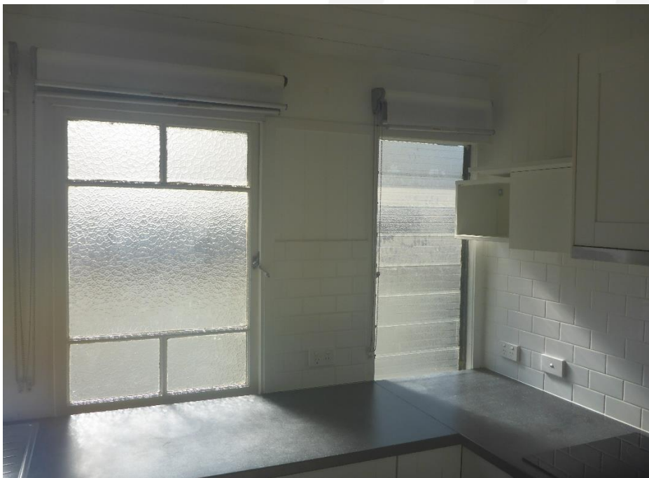
Figure 48: The reverse view within the kitchen space of the Unit 1 tenancy showing the mixture of original / traditional and contemporary windows that have been integrated into this section of the side verandah enclosure. (Source: VAULT)
