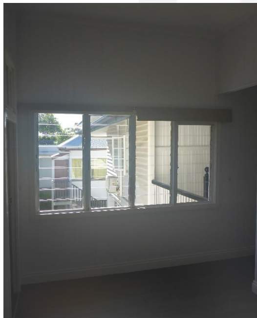
Figure 22: An internal view from the rear flat tenancy showing the later infill panel (with glass louvres etc.) as previously shown above at Figure 20 , which confirms that the enclosure of an open verandah walkway and integration of same into this rear tenancy (Unit 6). (Source: VAULT)
