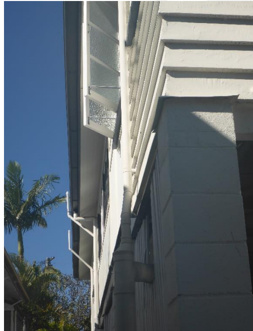
Figure 13: The view from the rear corner of the building looking forward along the northern (side) elevation of the subject heritage residential building, “Mimosa”. This side of the building was originally an open verandah return but has subsequently been fully enclosed as additional habitable space. (Source: VAULT)
