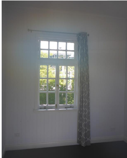
Figure 27: Another view from within the bedroom space of Unit 6 showing the original window assembly within the southern side wall – also refer to Figure 6 (above), intact interior wall construction etc. (Source: VAULT)
