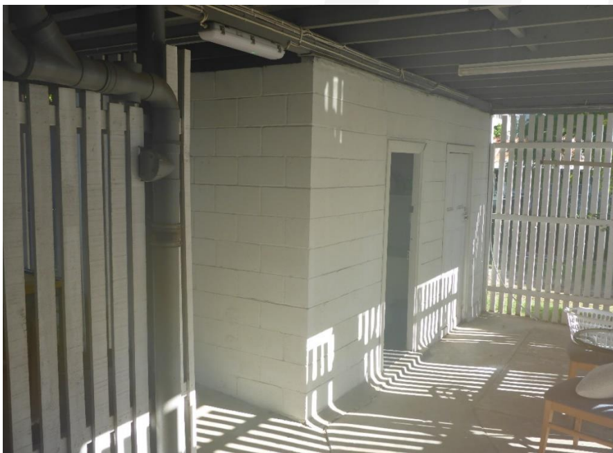
Figure 72: The undercroft space beneath the heritage residential building also incorporates a more contemporary laundry enclosure that has been constructed with concrete blockwork. (Source: VAULT)
