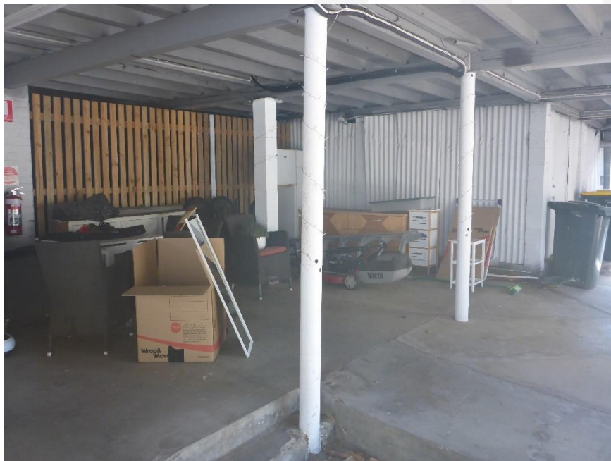
Figure 68: A broader view across the extant undercroft space beneath the heritage building, which shows the varied array of non-original support structures (i.e. steel posts or concrete columns) that are extant within this space. (Source: VAULT)
