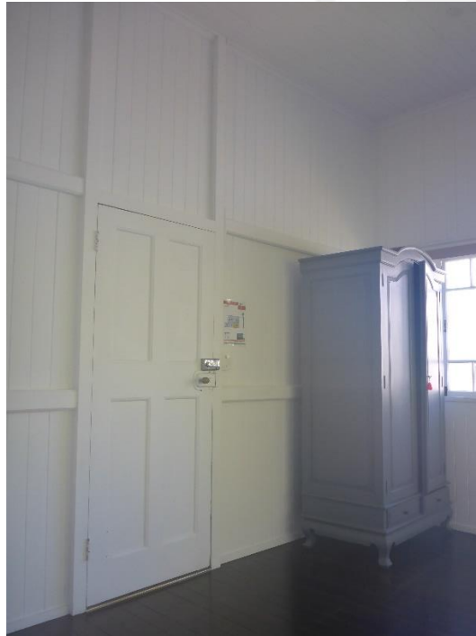
Figure 55: Another interior view from within the bedroom of Unit 2 showing the single skin construction of the infill wall that has enclosed this part of the original front verandah and the entrance doorway set within same. (Source: VAULT)
