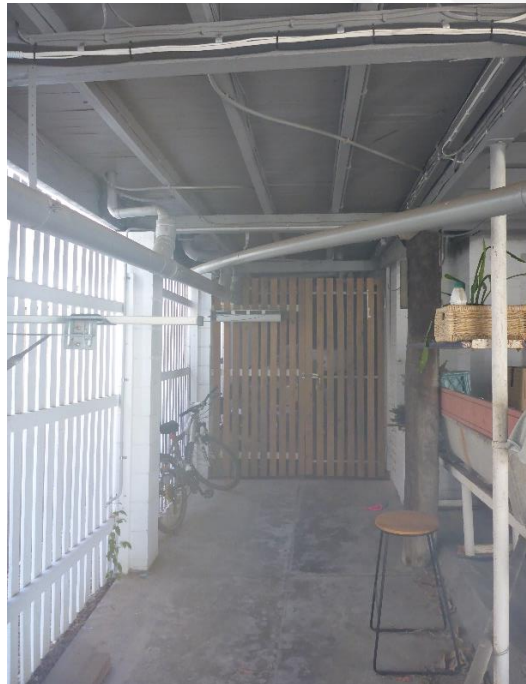
Figure 67: The view through the undercroft space extant beneath the side verandah enclosure situated along the northern side of the building core. The differential in sub-floor framing direction between the core of the building and the side verandah is readily identifiable in this image. (Source: VAULT)
