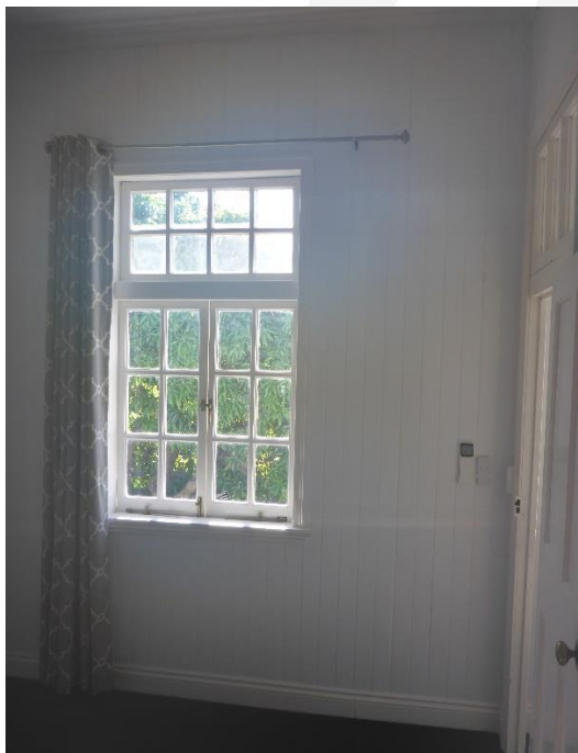
Figure 26: Another view from within the bedroom space of Unit 6 showing the original window assembly within the side wall – also refer to Figure 11 (above), intact interior wall construction etc. (Source: VAULT)
