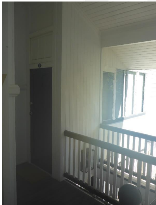
Figure 18: The view looking through the rear verandah space and showing the raked and timbered soffit of the roof overhand (at image top right) and the original timber balustrading of the access staircase. (Source: VAULT)
