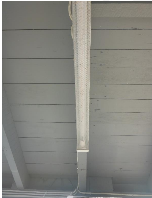
Figure 75: Another detailed view of the differentiation in floor lining that can be readily observed from within the undercroft space showing the wider gauge of interior timber flooring (at image left) and the narrower and lower grade species of the decking boards used where the original verandah spaces have subsequently been enclosed (at image right). (Source: VAULT)
