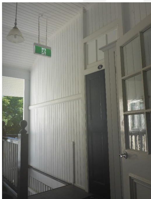
Figure 36: The view towards the entrance into Unit 5 from within the rear verandah space, which shows the intact wall construction and doorway assembly that leads into that rear flat tenancy. (Source: VAULT)
