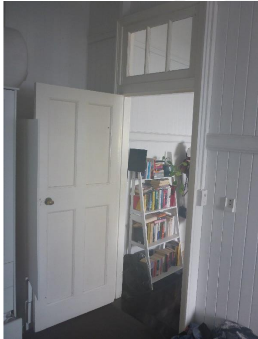
Figure 65: The reverse interior view from Figure 62 (above), which shows the original/ intact door and top light assembly within Unit 4 as viewed from within the bedroom space and looking through to the living area within that tenancy. (Source: VAULT)
