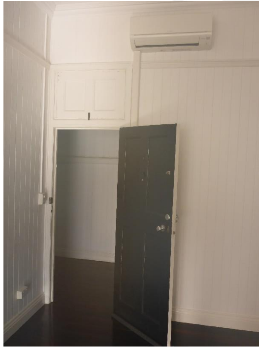
Figure 43: An interior view of Unit 1 showing the original doorway assembly located in the corner of the living space of that tenancy. (Source: VAULT)
