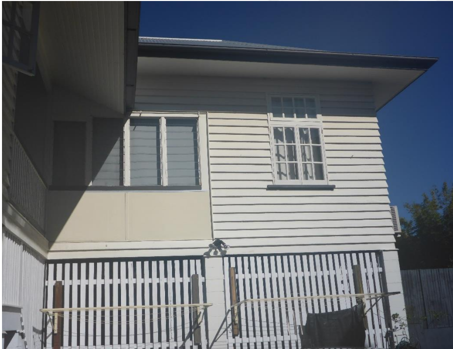
Figure 11: A more detailed view of the internal elevation of the rear Kitchen wing, which shows the more recent enclosure of what was originally an open verandah connection into that Kitchen wing. (Source: VAULT)
