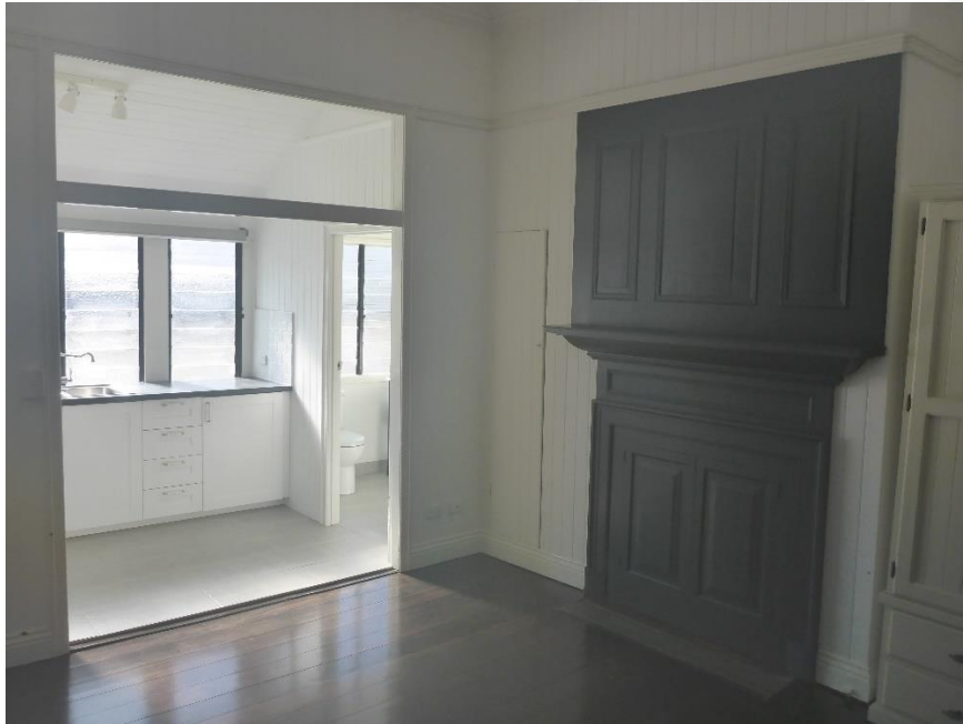
Figure 37: An interior view of Unit 3 showing the intact fireplace assembly (with enclosing panel over fireplace) and showing the removed French door assembly (at image left) that connects this core space with the enclosed verandah beyond and the kitchen installation integrated into that space. (Source: VAULT)
