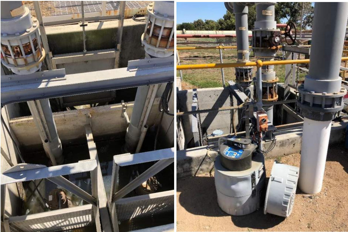
Figure 1.3 Drain 1 stormwater pit – capturing runoff from operational areas
