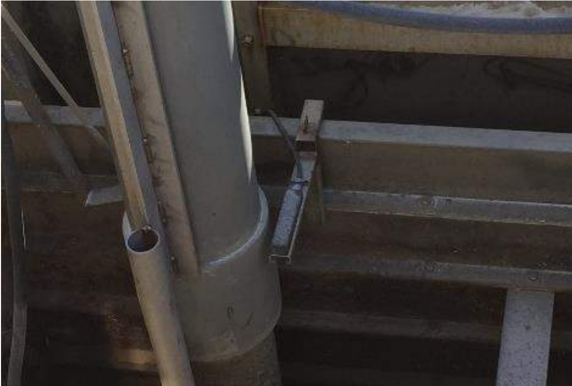
Figure 2.2 Flow meter installed at top of overflow weir
